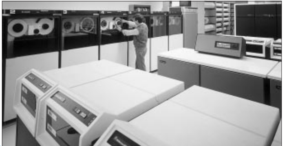
fig. J2-13: for large computer installations, the UPS cabinets are generally located in the computer room.
