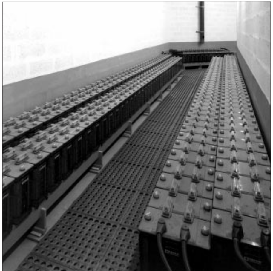
fig. J2-15: a typical battery room.
