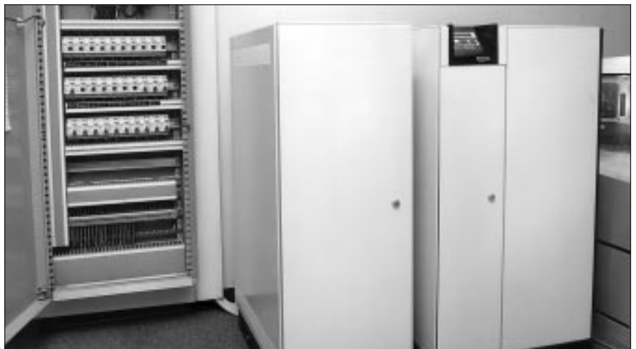
fig. J2-14: large UPS systems are frequently located in an electrical services room.
