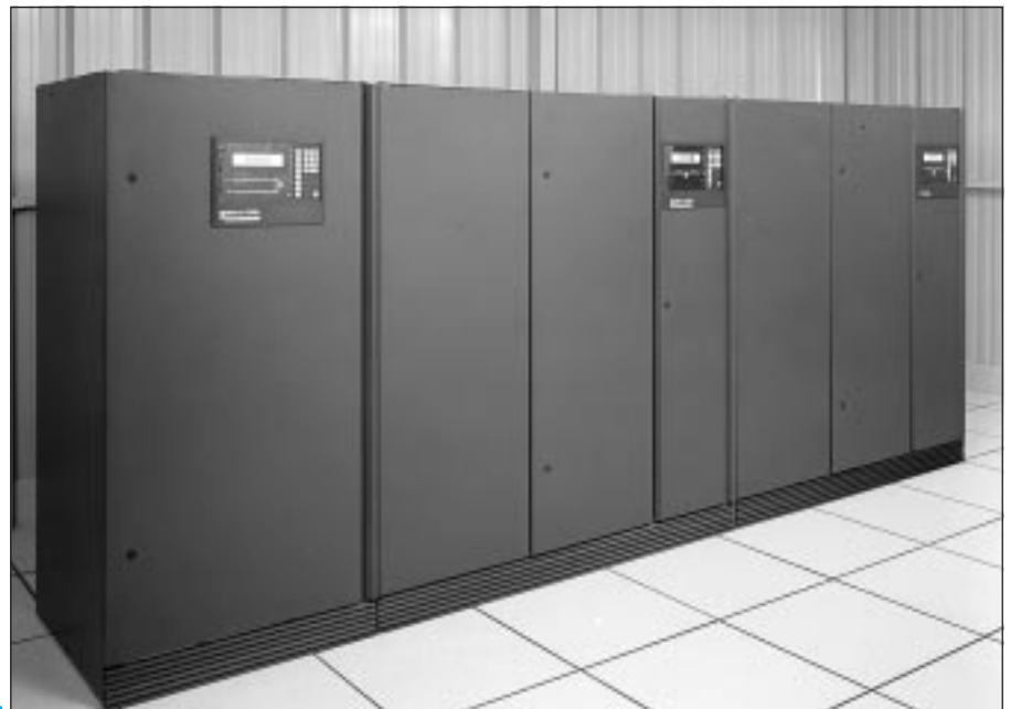
fig. J2-27: a UPS installation with incorporated communication systems.
